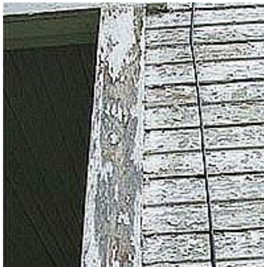
Paint Peeling on a House
